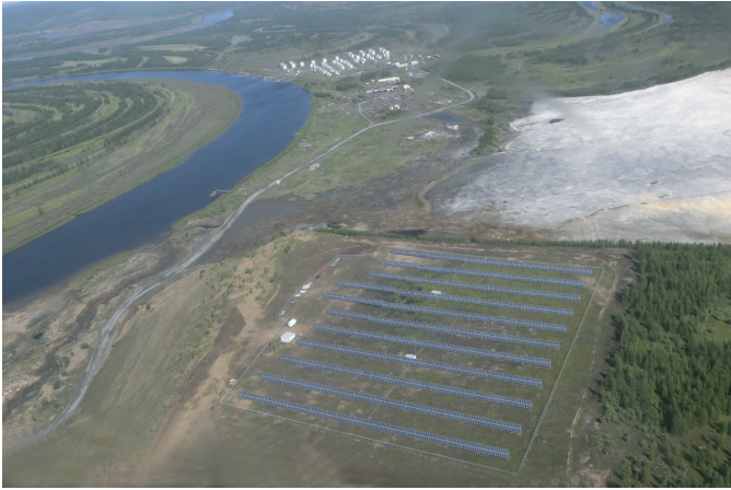
Illustration: Batagay solar power plant, the largest solar power plant north of the Polar circle. Capacity: 1 MW. Area size: 4.2 hectares. Equipment: Suntech STP300-24/Ve. Temperature range: max. +40°C, min. -45°C.
